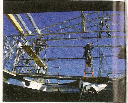
It is easy to frame barrel ceilings, domes and other details with steel.
